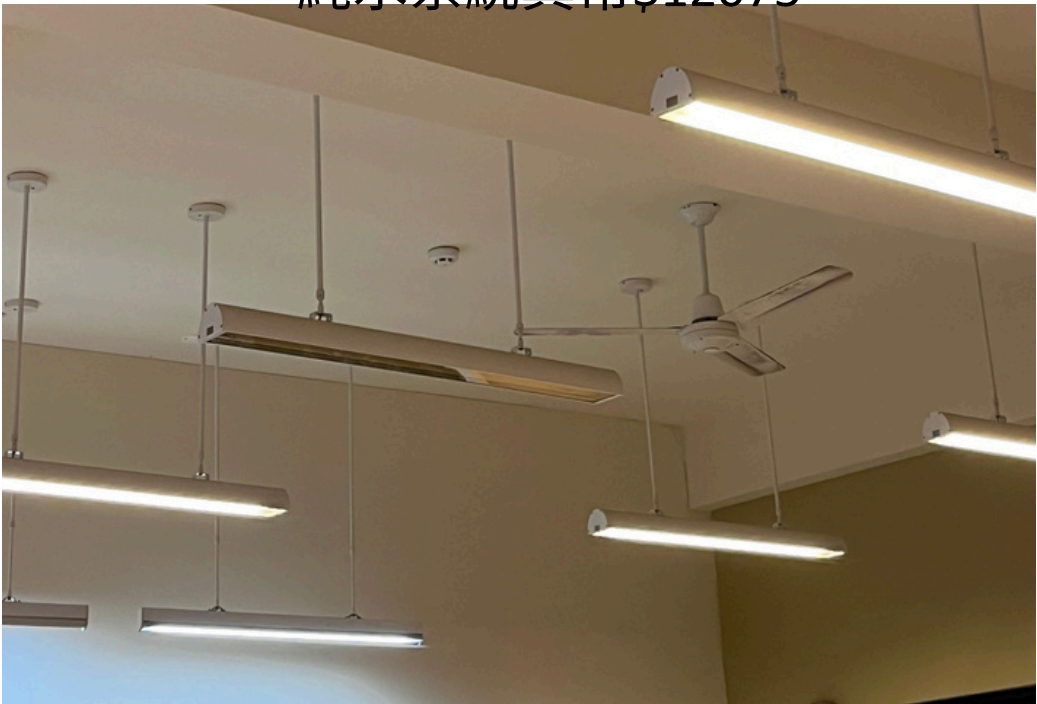
吊燈電源異常$2835
