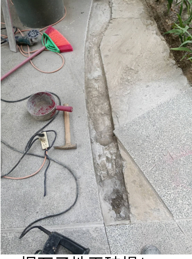
抿石子地平破損$5250
